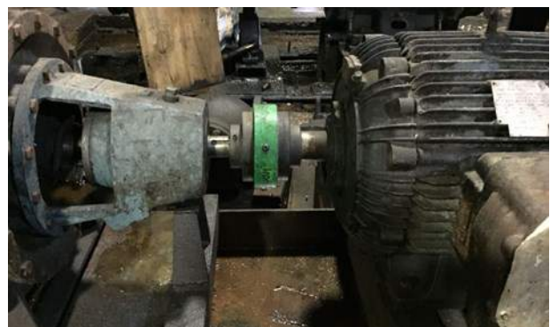
Centrifugal pump for general service
